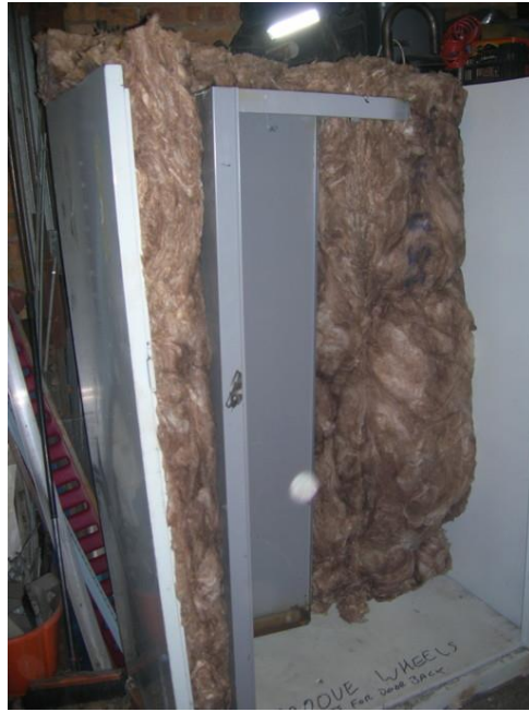
Overdid the insulation here, ended up using half this thickness all round
